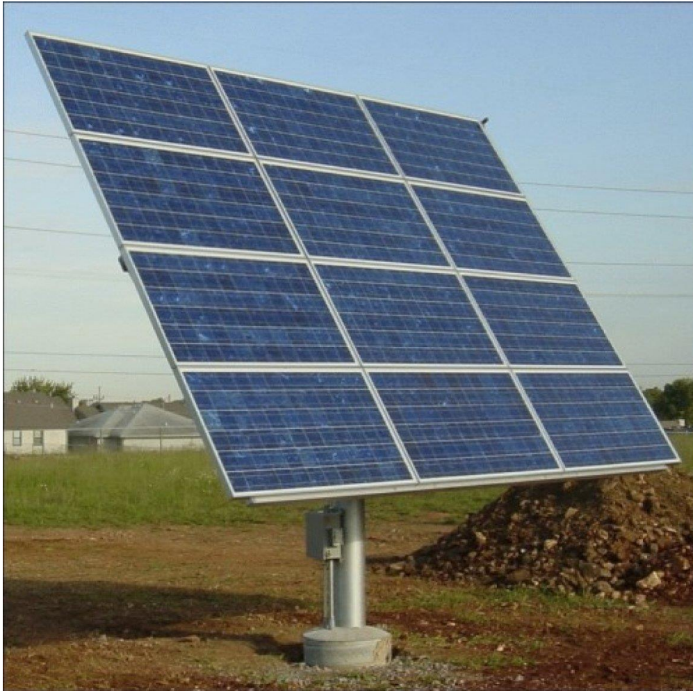
Figure: A PV tracker system, source: https://www.greentechrenewables.com/article/pros-and-cons-solar-tracking
