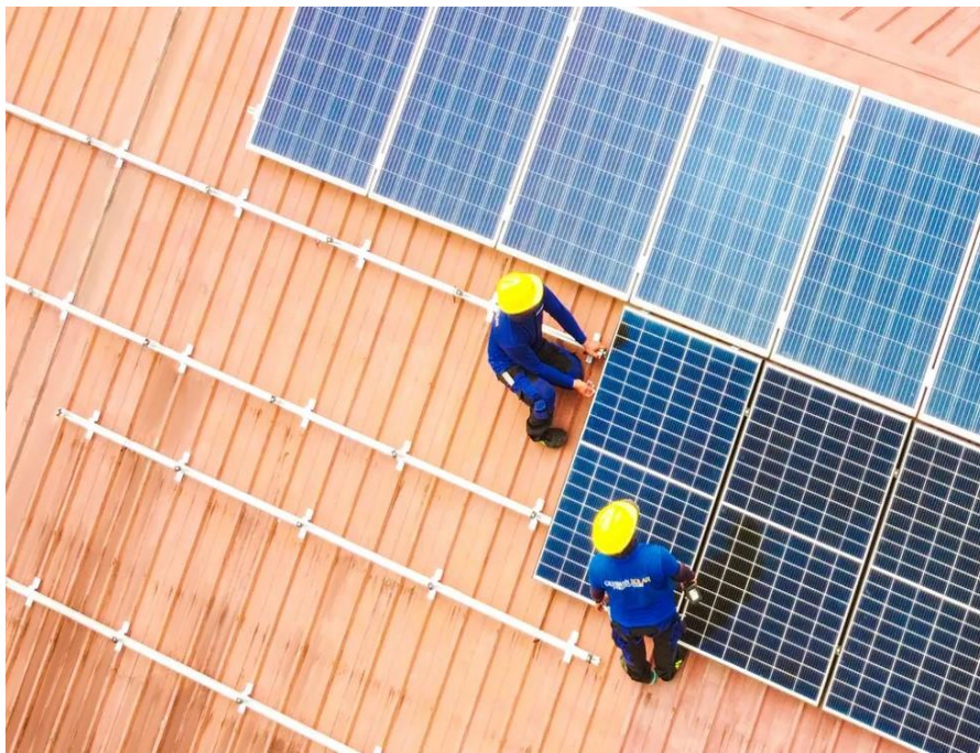
Figure: A installation of a photovoltaic system. source: https://www.philergy.com/post/is-my-roof-compatible-with-solar-panels-mounting-solutions-on-various-roof-materials-philergy
