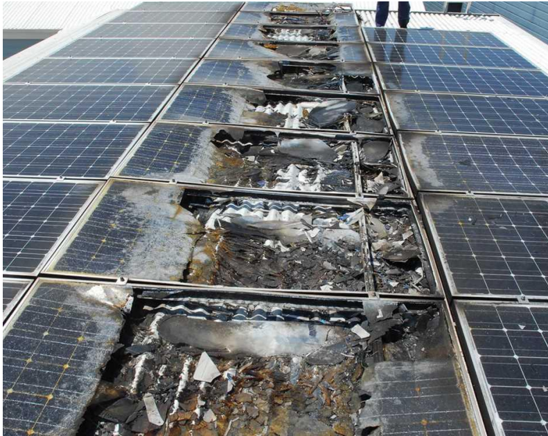
Figure: Solar installation under fire , source: https://www.pv-magazine.com/2021/07/02/australias-unsafe-solar-installation-standards-under-fire/
