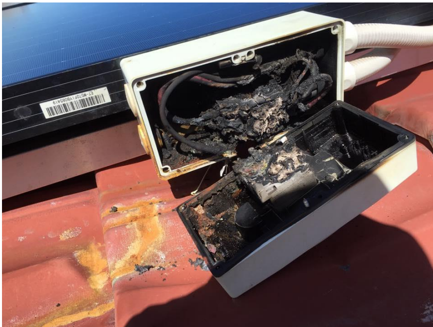
Figure: Poor quality junction boxes with unstable cable connections are potential points of arcing fault occurrence.
