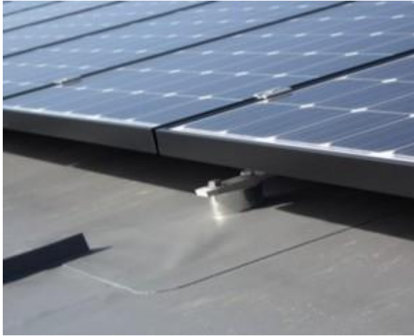
Figure: One engineering solutions for fixing PV arrays on flat roofs, source: https://www.singleply.co.uk/fixing-solar-panels-to-flat-roofs-why-we-recommend-an-engineered-solution/
