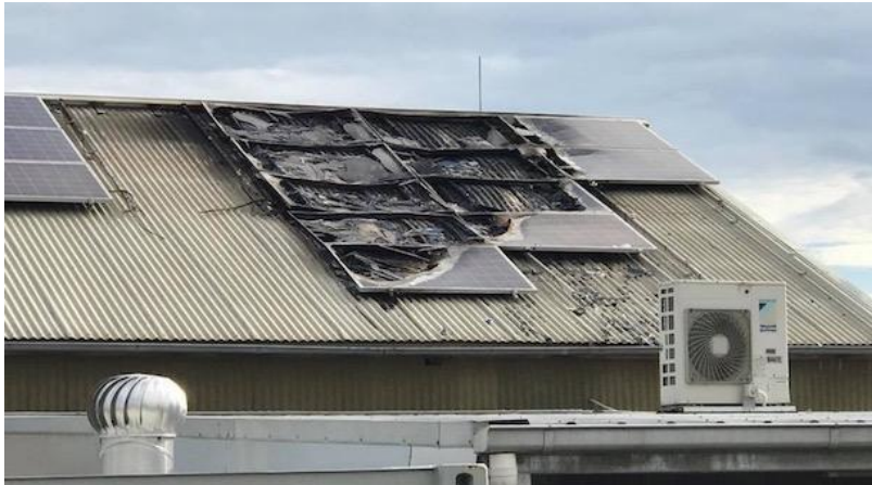
Figure: Fire caused by DC arcing
