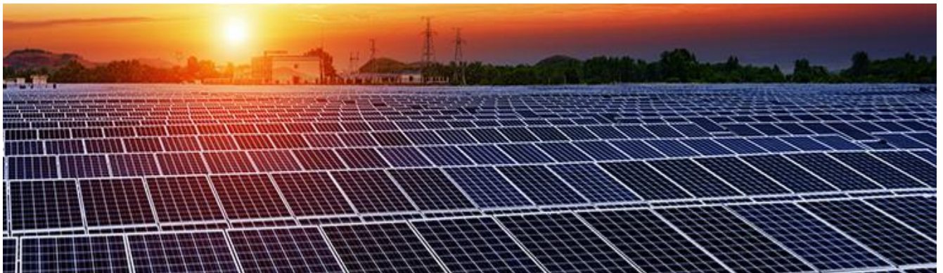
Figure: The quality and successful operation of a PV system depends on its proper organization and management. source: https://www.intertek.com/solar/
