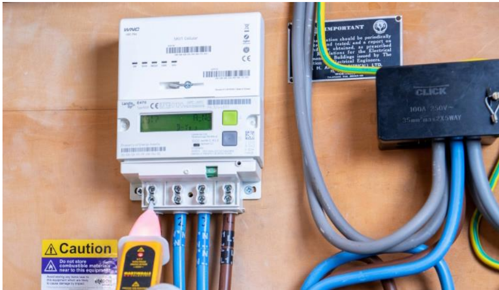
Figure: A smart meter, source: https://www.smartestenergy.com/en_gb/business/smart-meters/
