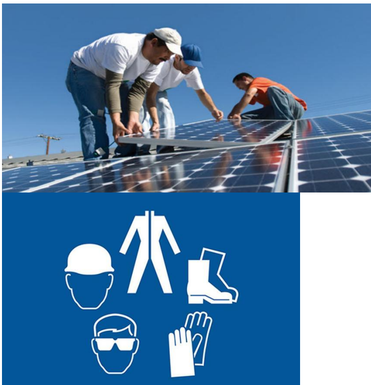
Figure: Installers of PV Systems and safety risks,
