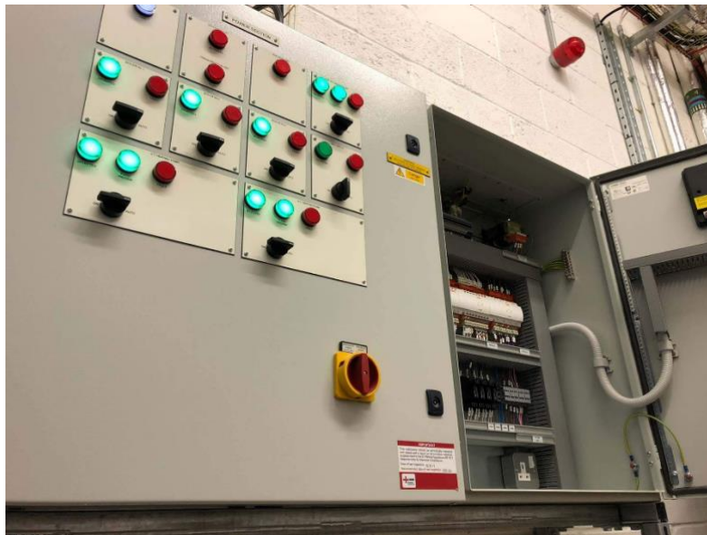
Figure 16 Control unit of a Building Management System
