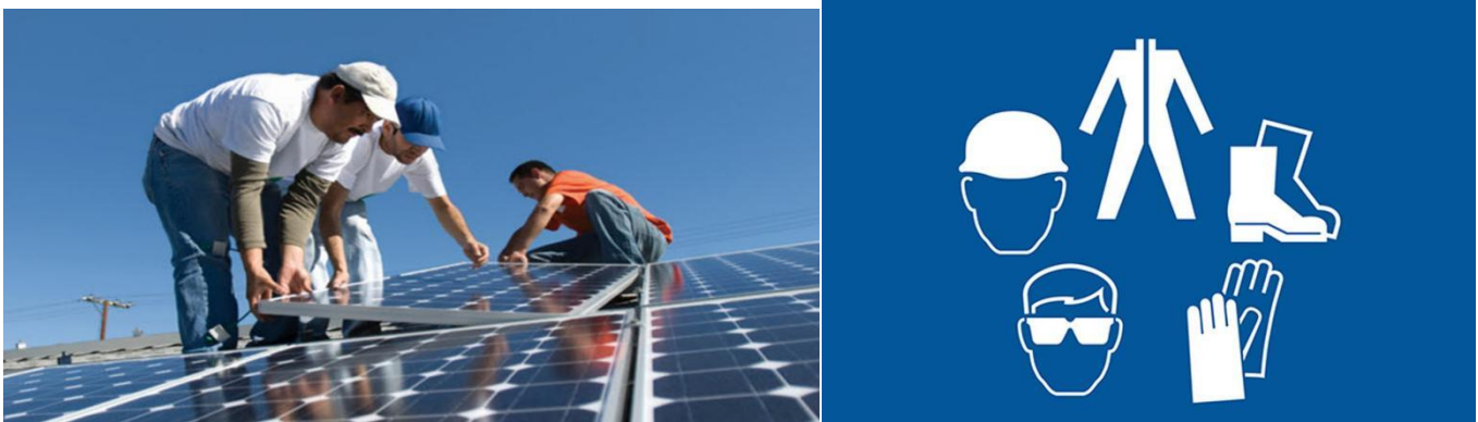
Figure: Installers of PV Systems and safety risks , source: https://www.thehartford.com/insights/home-workplace-safety/solar-energy-benefits-safety-risks
