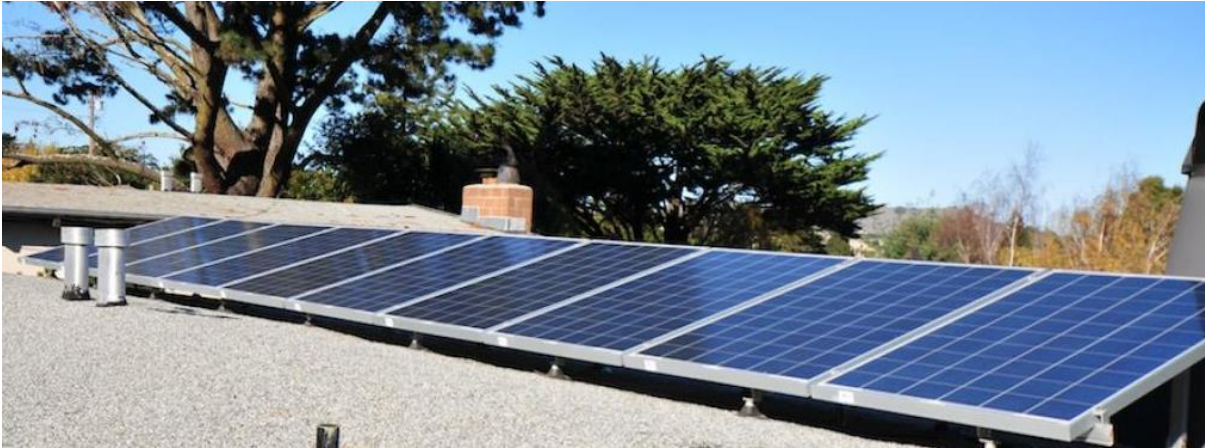
Figure: PV system on a one tar and gravel roof , source: https://www.greentechrenewables.com/customer-project/235kw-sunny-sausalito-ca-solar-install
