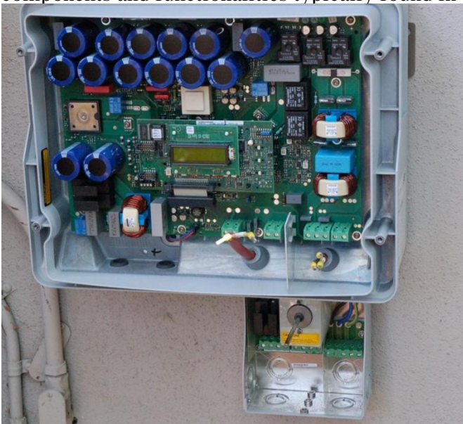
Figure: A photo of the device and elements of an inverter. source: https://sinovoltaics.com/learning-center/inverters
