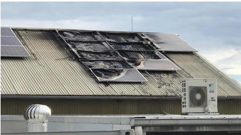
Figure: Fire caused by DC arcing faults, source: https://www.acsolarwarehouse.com/news/solar-fires-dc-arc-faults-on-solar-systems/
