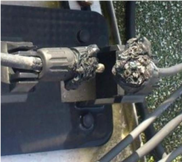
Figure: A cross-mating connectors from two different manufacturers potential points of arcing fault occurrence.
