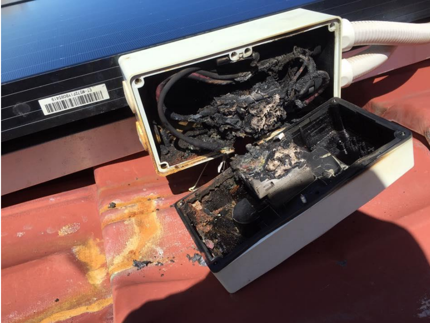
Figure: Poor quality junction boxes with unstable cable connections are potential points of arcing fault occurrence.
