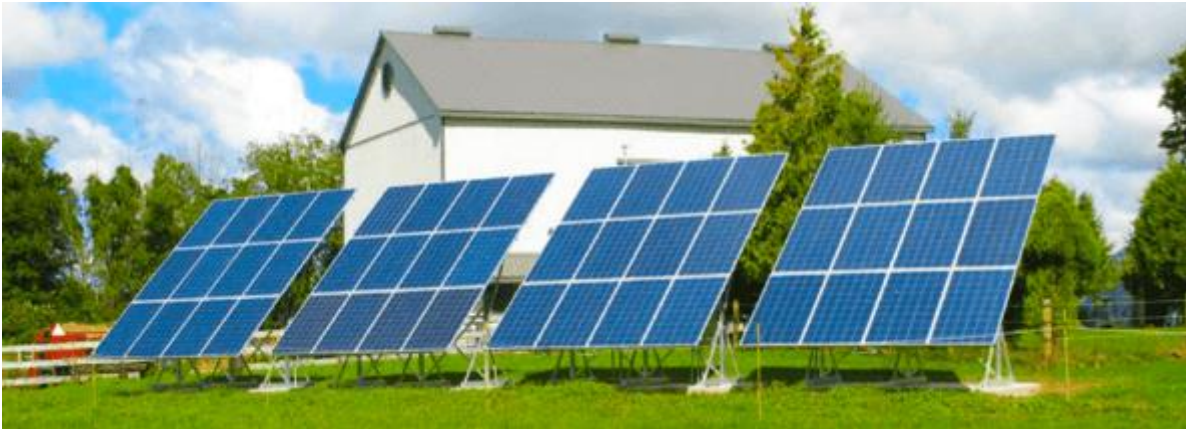
Figure: Ground Photovoltaic System , Source: https://news.energysage.com/ground-mounted-solar-panels-top-3-
