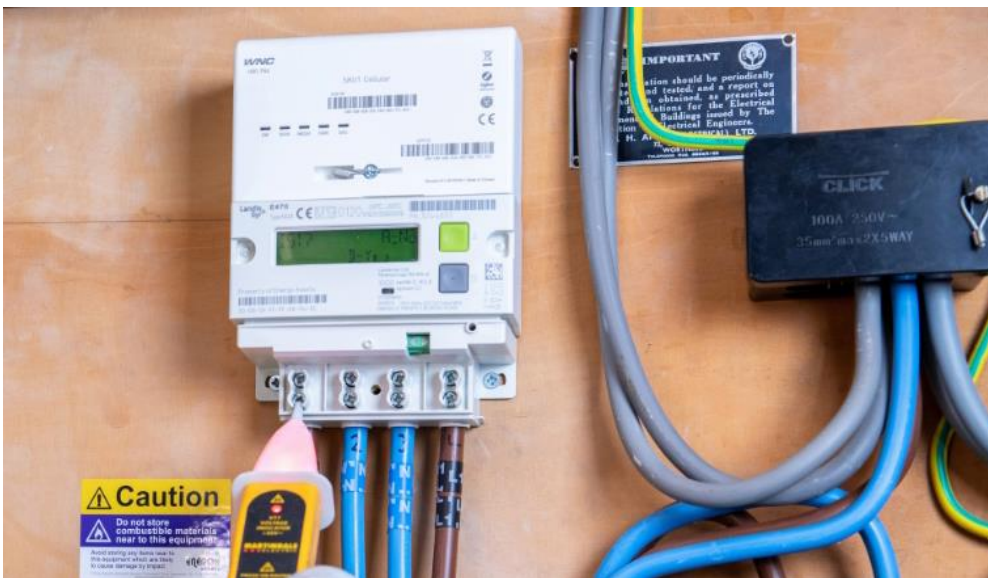
Figure: A smart meter , source: https://www.smartestenergy.com/en_gb/business/smart-meters/
