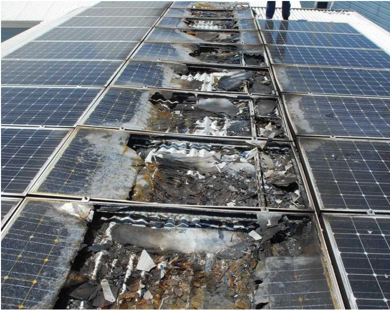
Figure: Solar installation under fire , source: https://www.pv-magazine.com/2021/07/02/australias-unsafe-solar-installation-standards-under-fire/
