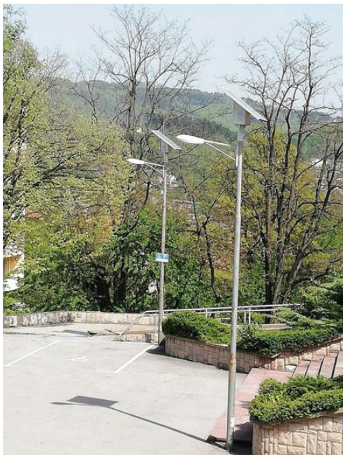
PV–LED outdoor lighting
