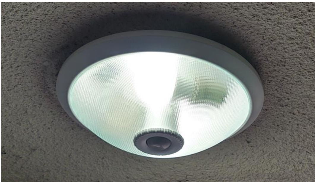
4.10. Luminaires with a built-in infrared sensor
