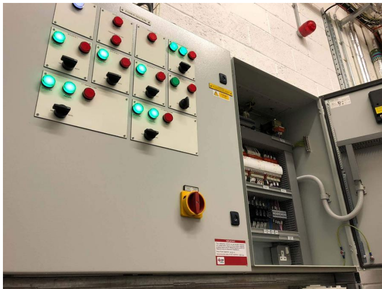
Figure 16 Control unit of a Building Management System
